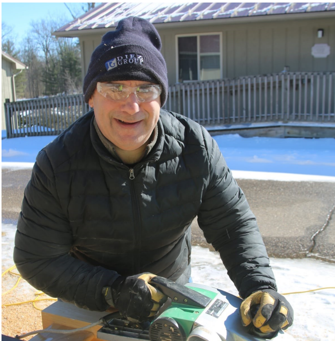
ZC Jim Diez works to trim the bunkbed frames down just enough to make them fit back into their spaces more easily.
