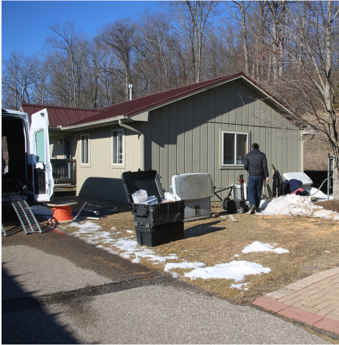
Browning Power Systems worked to install a new 22KW generator for the cabins.
